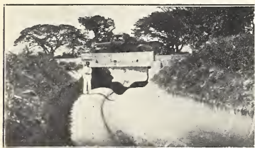
FIG. 6. Maracay, Venezuela. This large collecting ditch was lined with three rows of third rounds of pipe 36 inches in diameter, two rows of sixth rounds of pipe 36 inches in diameter, two rows of flat slabs 16 inches by 24 inches.
